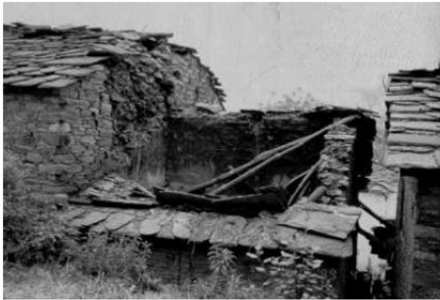
Figure 21 Roof collapse due to lack of anchorage
