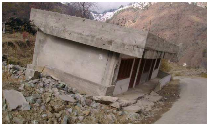
Figure 50 Building constructed on unlevelled foundation leading to its settlement
