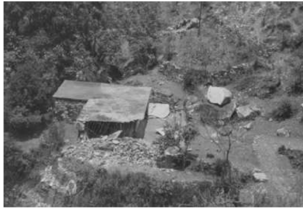
Figure 14 Building damage due to rock fall
